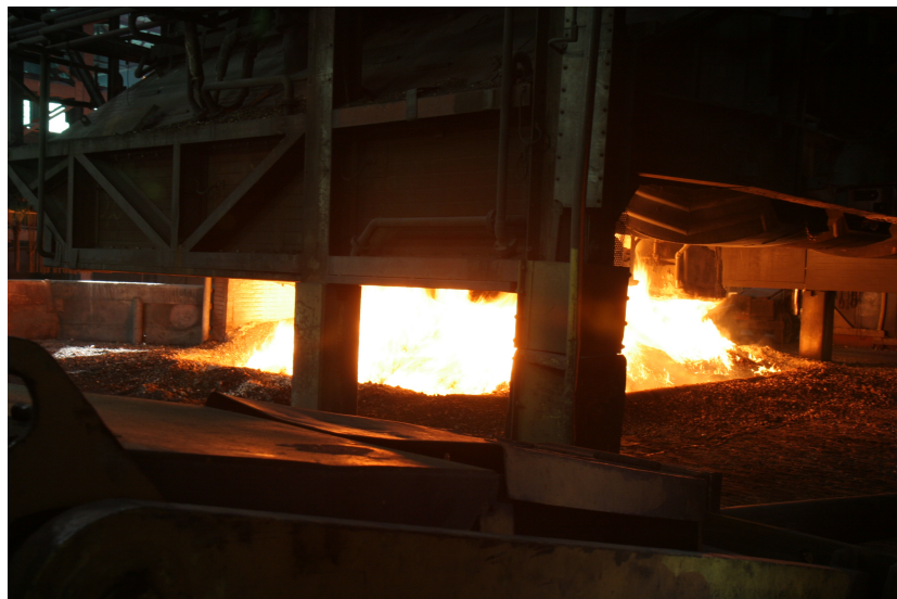
Submerged Arc Electric Furnaces
